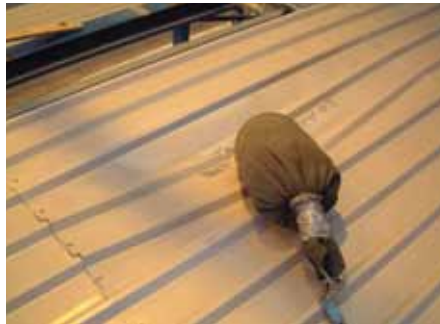
Figure 6. Successful non-fragility test with minimal damage on nominal 0.7 mm gauge liner
