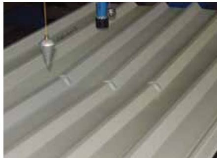
Figure 9. Failed pre-finished steel profiled sheet showing local buckling
