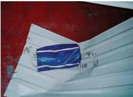
Figure 5. Failed non-fragility test where fasteners have torn through and the sheeting has failed
