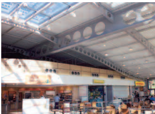
Structurally efficient cellular beams used to create flexible, column-free space at this motorway service station.
