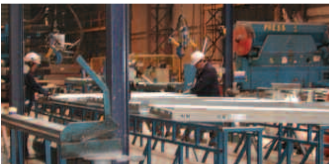
Factory assembly of steel construction components. Off-site manufacture is more efficient, faster, leaner and safer than site construction.
