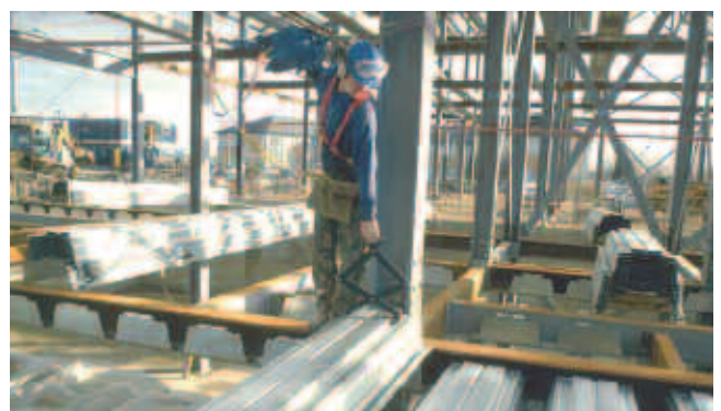
Installing 'deep' steel decking on the lower flanges of asymmetric Slimflor® beams.
