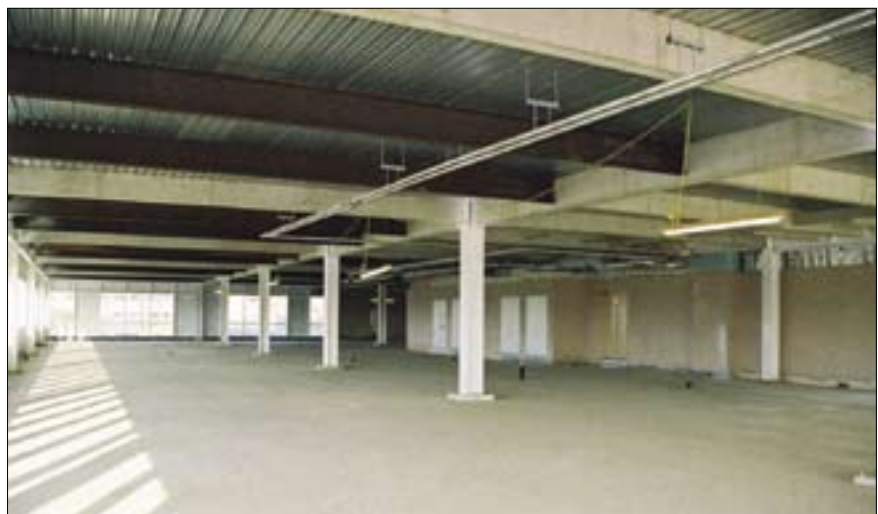
Figure 61 T-Mobile HQ, Hatfield. Use of Fire Safe Design led to unprotected secondary beams and significant economies in fire protection costs.
