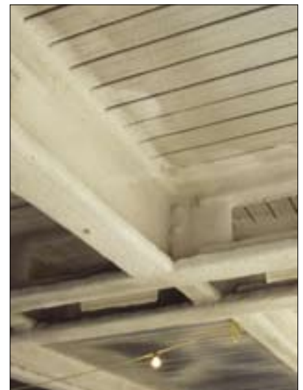
Figure 24 Spray protection system.
