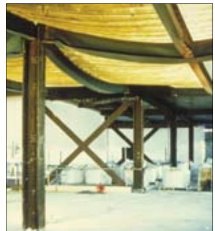
Figures 57, 58, 59 Office fire loading supplemented with wooden cribs produced the most extreme temperatures in any of the six fire tests. Despite this, the unprotected steel beams (which reached temperatures in excess of 1100°C) and floor did not collapse.
