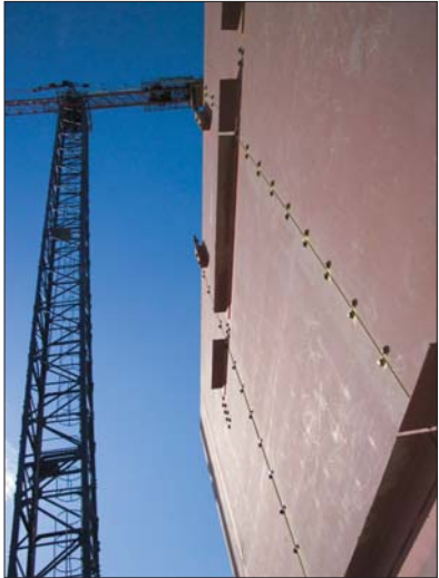
Left: Bolted together panels in the central core Far right: Architect's visualisation of finished project
