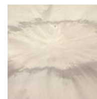
Above: Surface damage to reinforced concrete (top) and to Bi-Steel (bottom) after a close-in explosion
