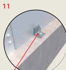
11 Angle welded to Bi-Steel panel to accept temporary holding down bolts cast into the foundation
