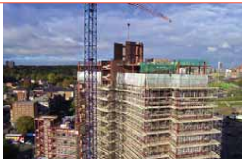
Above: Corefast - the future in building cores Left: Birmingham 1 - finished development and Corefast core under construction
